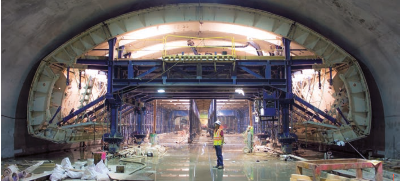
Second Avenue Subway in the making, New York, 2013. MTA Capital Construction/Rehema Trimiew/Wikimedia, © BY-SA
